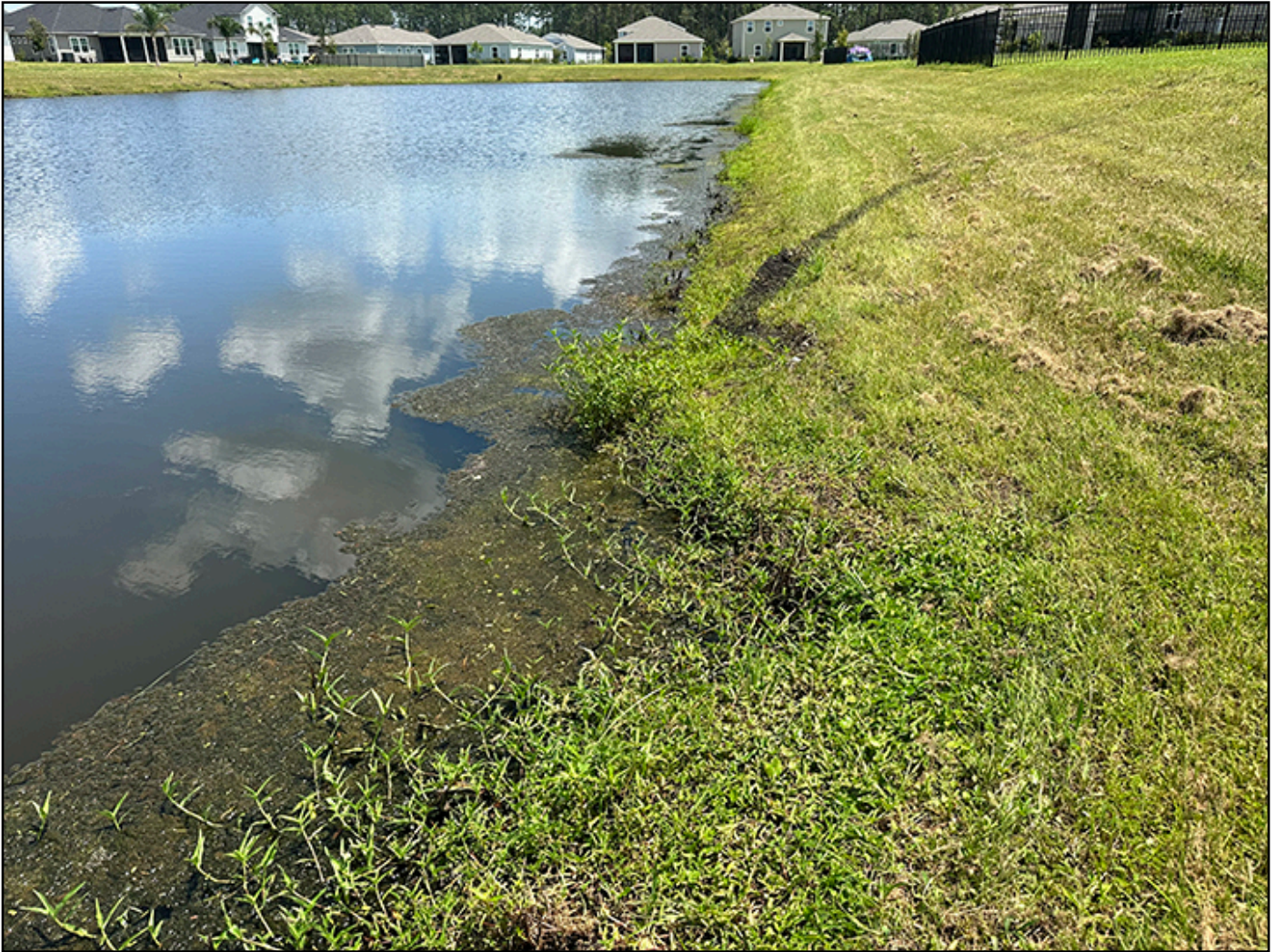
Figure No. 5 - Sector B radius exiting toward the South bank embankment loss.
