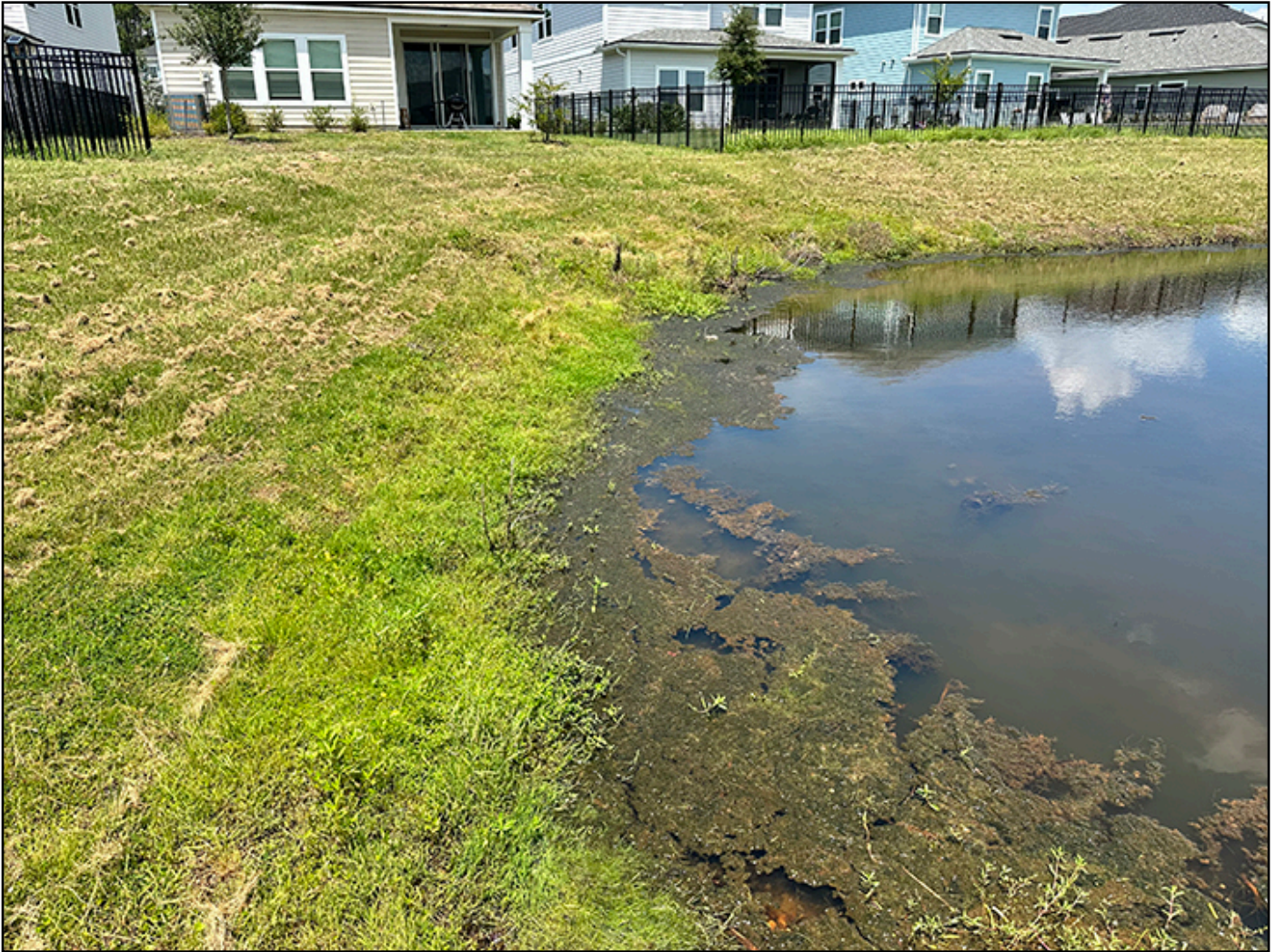
Figure No. 4 - Sector B embankment deterioration through the radius.
